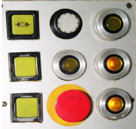
Figure 6: Poor or impermanent marking of a control panel
